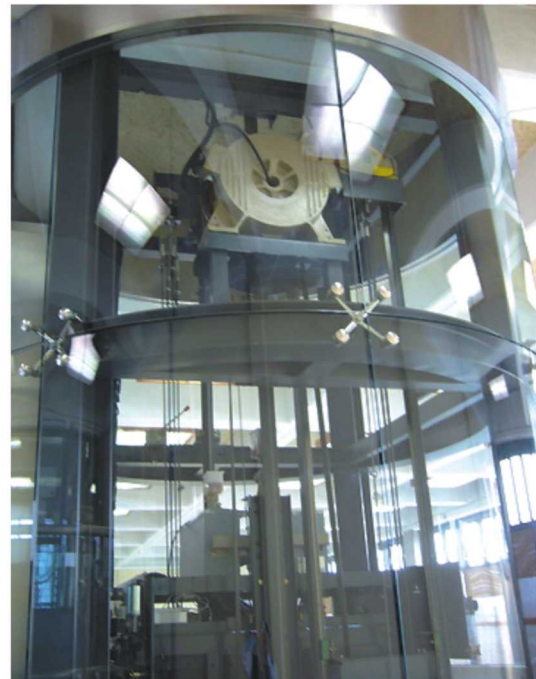
桃園國際機場第一航廈觀光梯，永磁同步無機房主機 Permanent magnet synchronous roomless winch of Taiwan Taoyuan International Airport terminal 1 tourist elevator.
